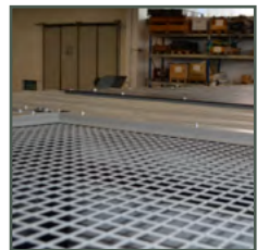
Air outlet louvres with metal mesh to protect the expulsion from leaves/dirt
